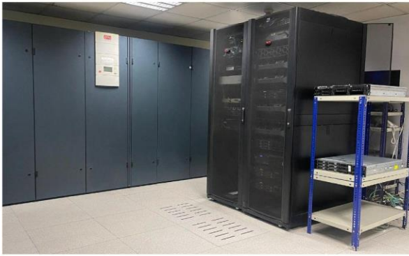
DATA CENTER HQ ML&C Rwp
